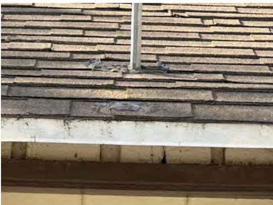
Detail at roof; note heavy tar/sealant around pipe penetration (ARG, 2023).
