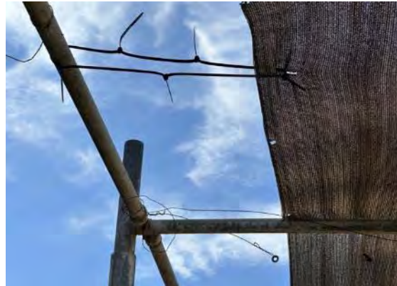
Detail at canvas awning; note tears and zip ties (ARG, 2023).
