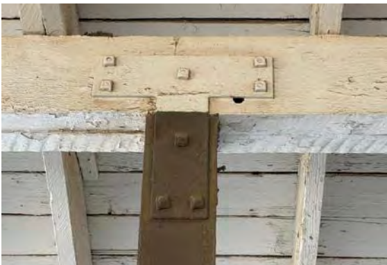
Detail at typical column/beam connection with T-shaped steel plates and bolts (ARG, 2023).
