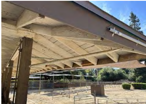
Detail at southwest corner of roof; note additional brace at overhang (ARG, 2023).
