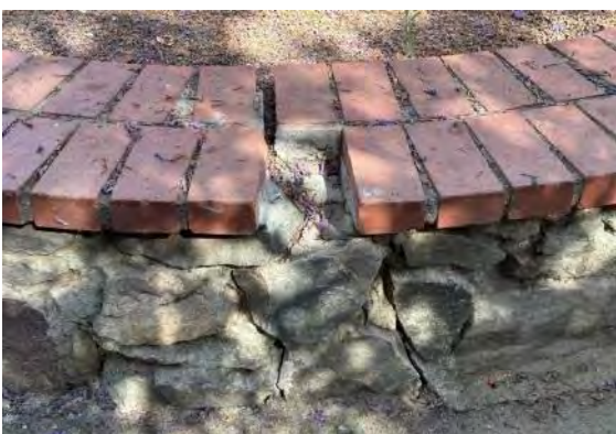
View of planter wall; note cracking and missing paver (ARG, 2023).
