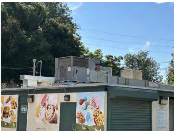
View of HVAC and kitchen equipment at roof (ARG, 2023).
