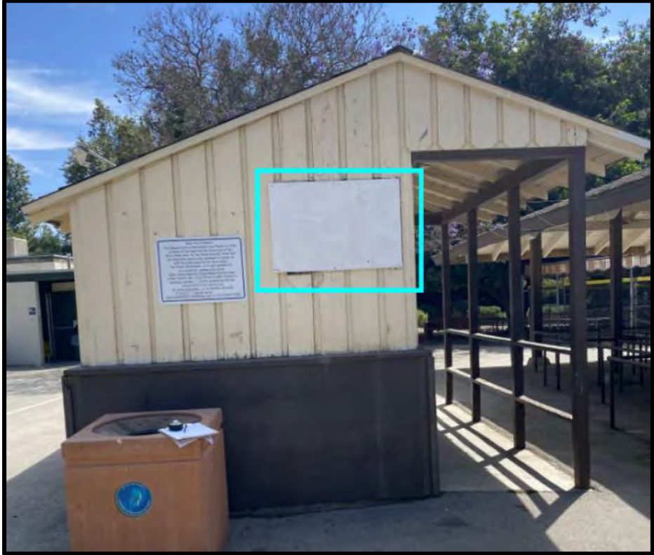
Figure 39 View of the improperly patched opening at the west wall of the Ticket Booth.
