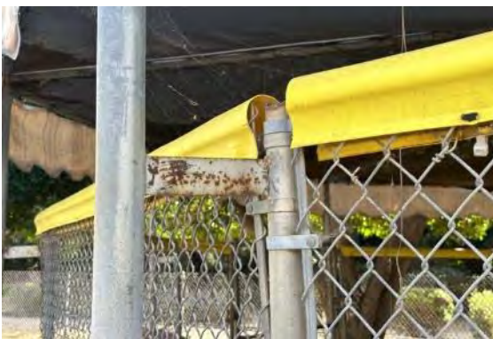
Detail at pipe framing and chain-link fence; note corrosion (ARG, 2023).
