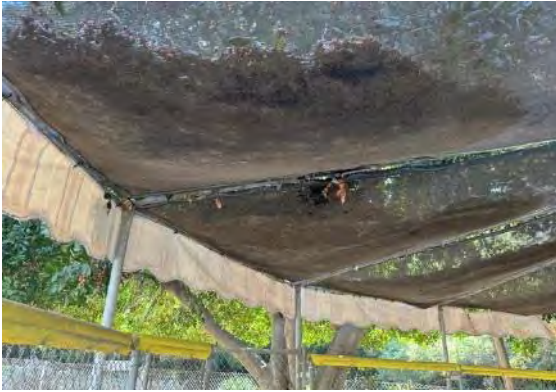
Detail at roof awning; note heavy collections of leaves/debris, and stained and sagging mesh panels (ARG, 2023).
