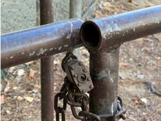
Detail at metal stanchions; note paint loss and missing end cap (ARG, 2023).
