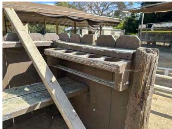
Detail of cup holders at stand; note termite damage at wood post (ARG, 2023).
