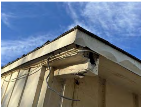
Detail at northeast corner of roof; note heavy wood rot at rafter tail and dented sheet metal edge flashing (ARG, 2023).
