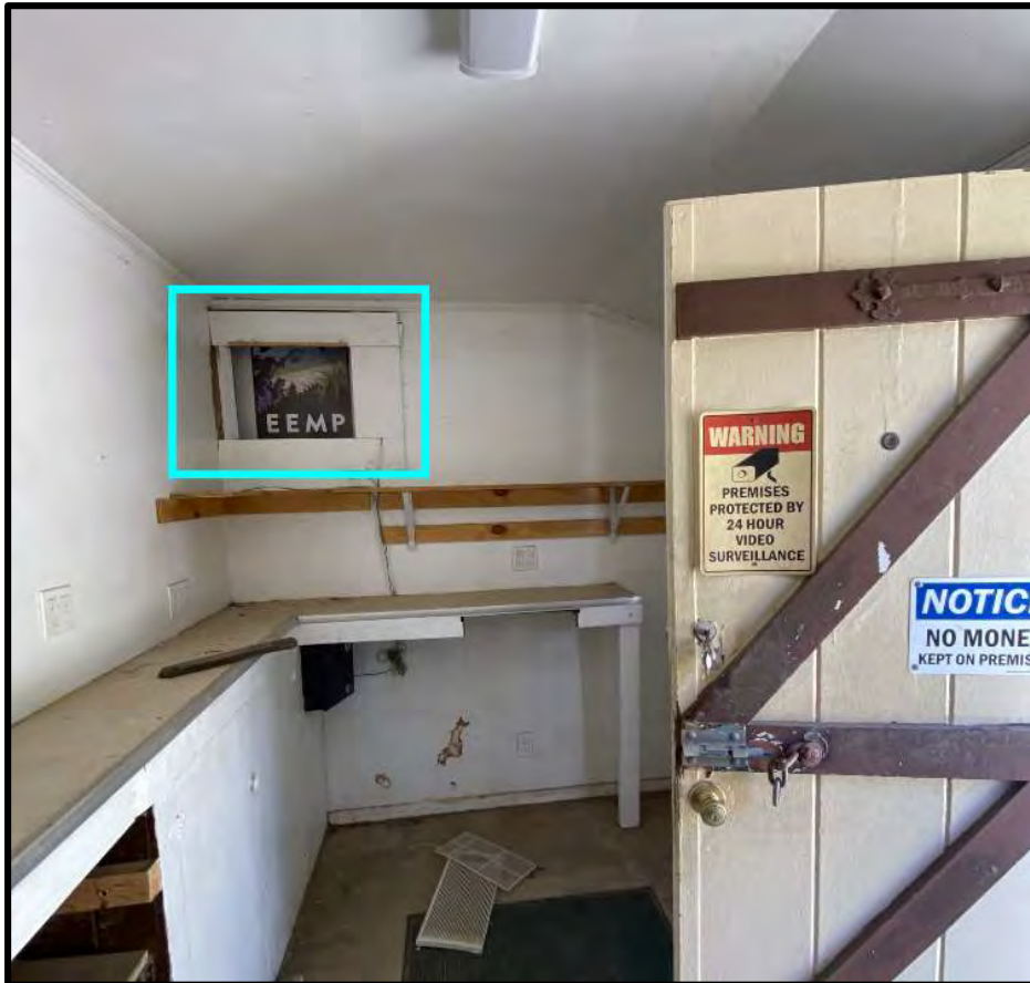
Figure 47 Interior view of the opening in the west wall of the Ticket Booth.
