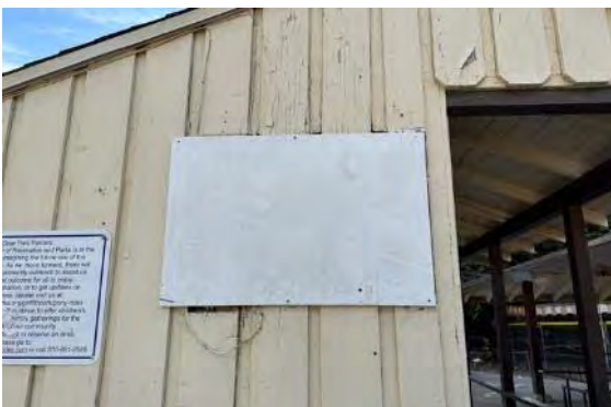
Detail at west façade; note infill panel covering hole for A/C unit (ARG, 2023).
