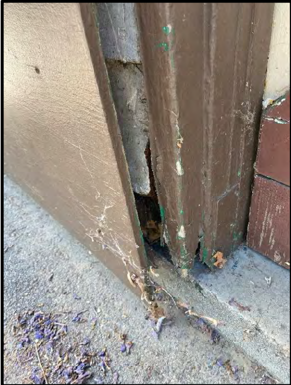
Figure 37 Close up of the deteriorated, original horizontal siding.
