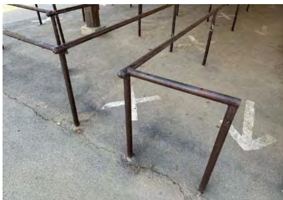
Stanchions and directional markings at asphalt pavement; note cracks and missing end cap (ARG, 2023).
