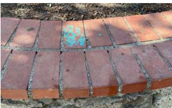
View of planter wall; note graffiti at brick paver (ARG, 2023).
