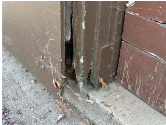
Detail at door frame; note heavy wood decay/loss at frame and wall (ARG, 2023).
