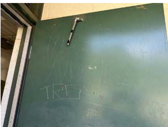
Detail of scratches at restroom door (ARG, 2023).
