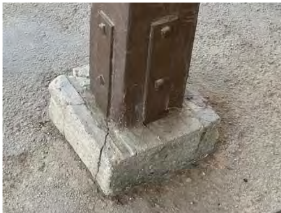
Detail at typical column base; note cracks in concrete footing (ARG, 2023).
