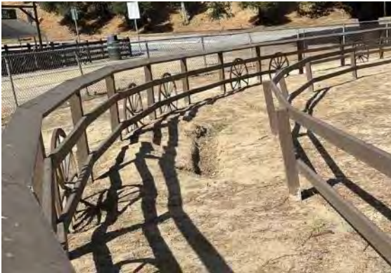
Deep rut at south end of riding ring (ARG, 2023).
