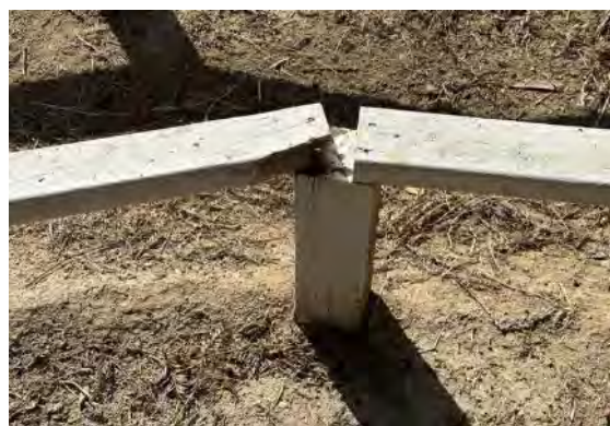
Typical splits and wood loss at guide rails/post connection (ARG, 2023).
