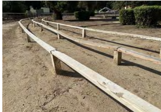
View of inner guide rails; note sagging rail (ARG, 2023).
