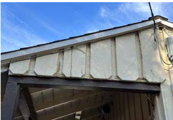
Detail at east façade over porch; note splits in vertical siding (ARG, 2023).
