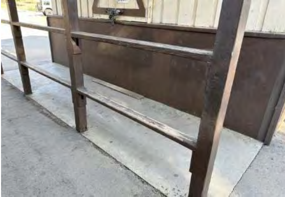
Porch railings; note heavy wear damage and paint loss (ARG, 2023).
