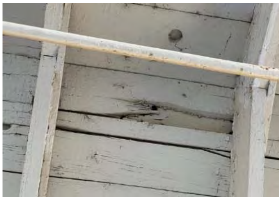
Detail of board sheathing; note splits, knotholes, and losses (ARG, 2023).
