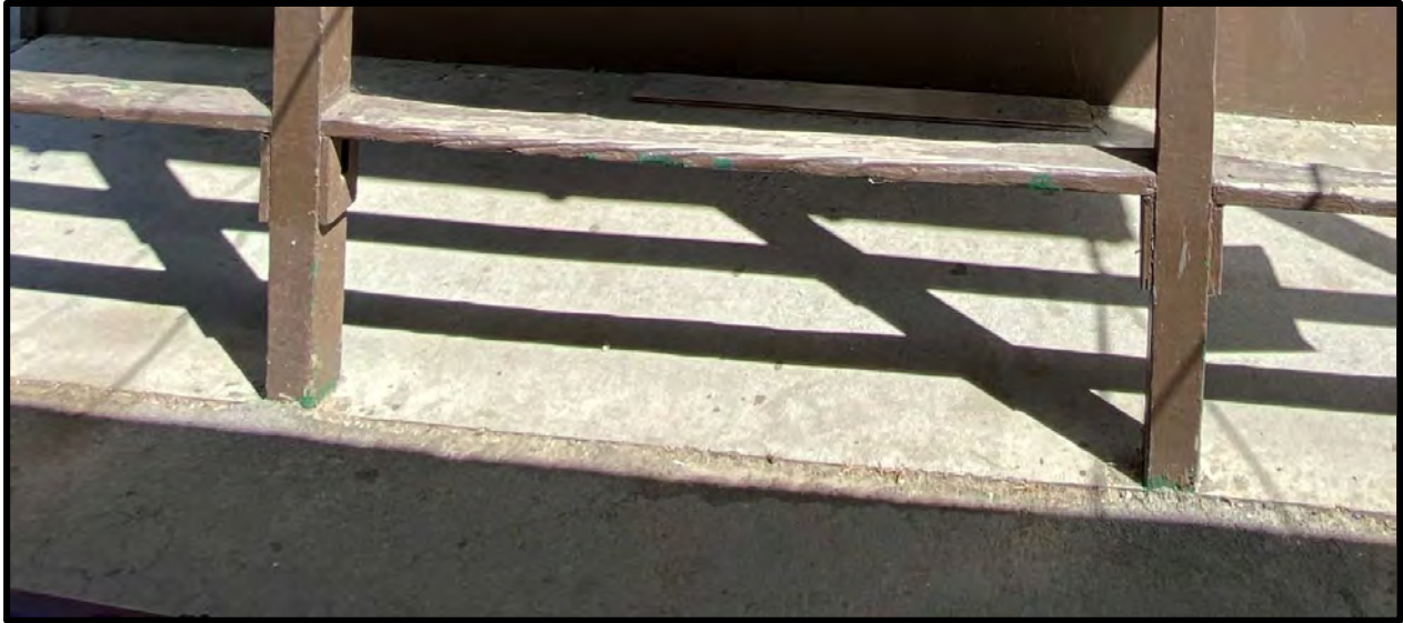
Figure 40 View of minor biological growth and insect damage at the base of the Ticket Booth columns.
