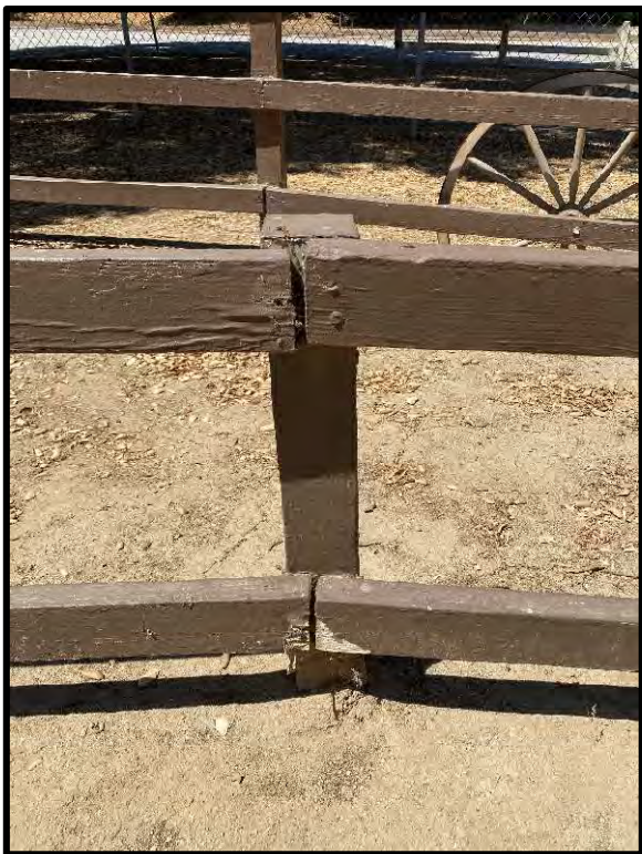
Figure 28 Close up of a Running Guide Rail post and rail.
