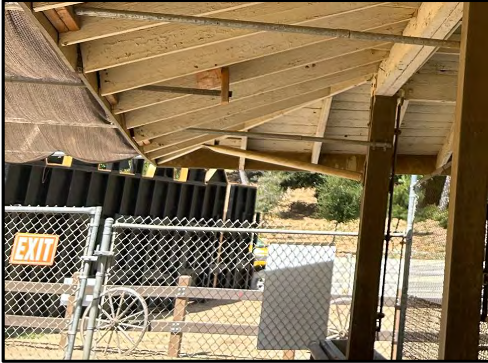
Figure 35 View of the Pergola roof corners deflecting.
