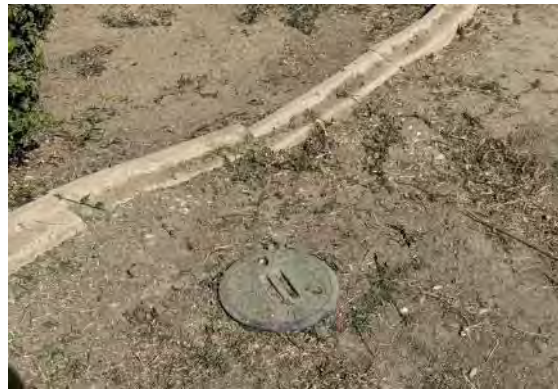
Detail of shifted curbs (ARG, 2023).
