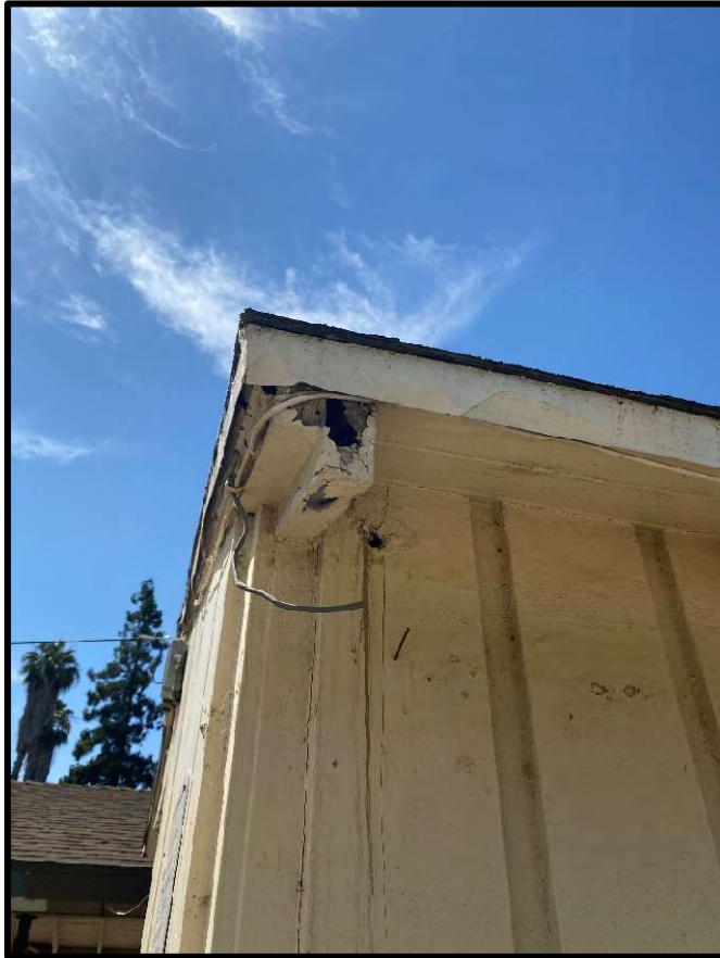
Figure 38 View of the roof rafter deterioration at the ends of the member.
