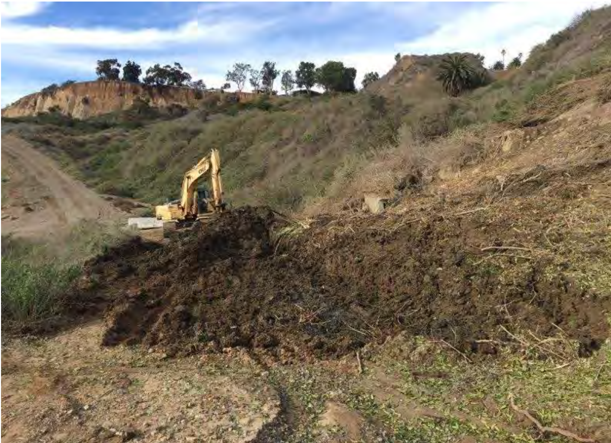
Photo 6: The Contractor excavated mud and debris, and placed geotextile on the roadway to allow safe passage from the project stockpile into the canyon and continue construction
