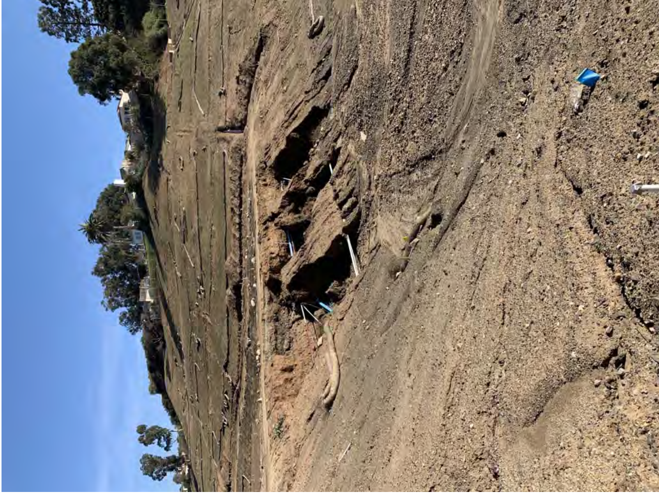
Photo 1: Looking northeast at the Basin 9 berm after the December storms. Severe erosion caused collapse of the berm and washed mud into the basin.
