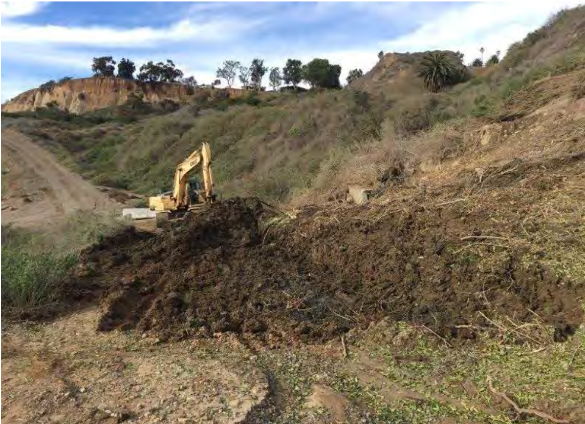
Photo 6: The Contractor excavated mud and debris, and placed geotextile on the roadway to allow safe passage from the project stockpile into the canyon and continue construction
