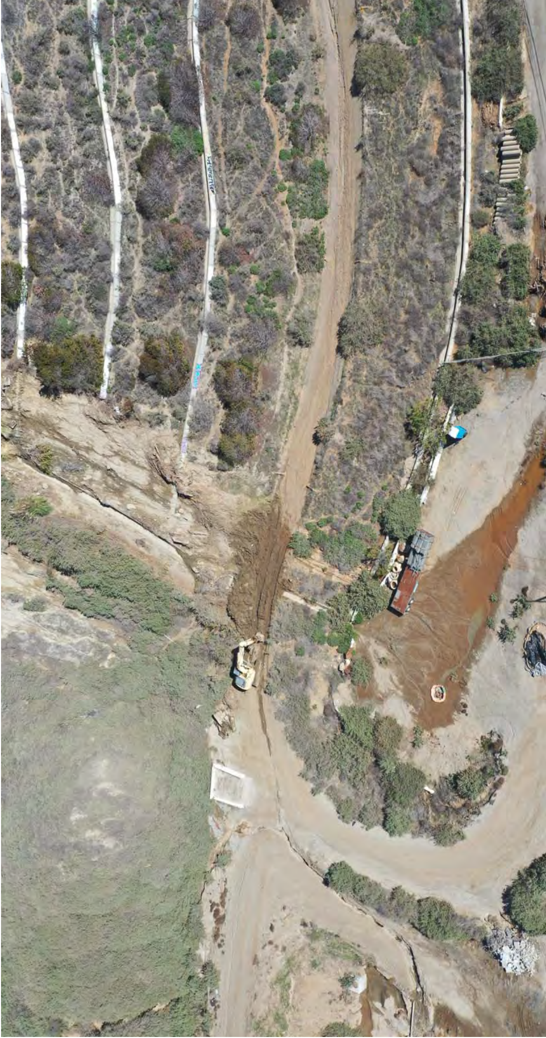
Photo 7: Looking northeast from Pacific Coast Highway. A landslide deposited mud and debris onto the access road. Severe erosional rutting also prevented access to the project stockpile as shown on the left.
