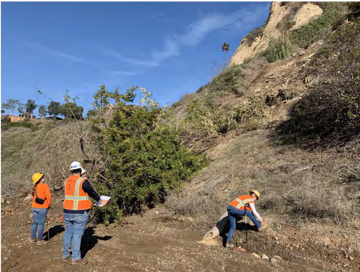
Photo 5: Looking northwest along the access road near PCH. A landslide deposited mud and debris, rendering the road impassable.
