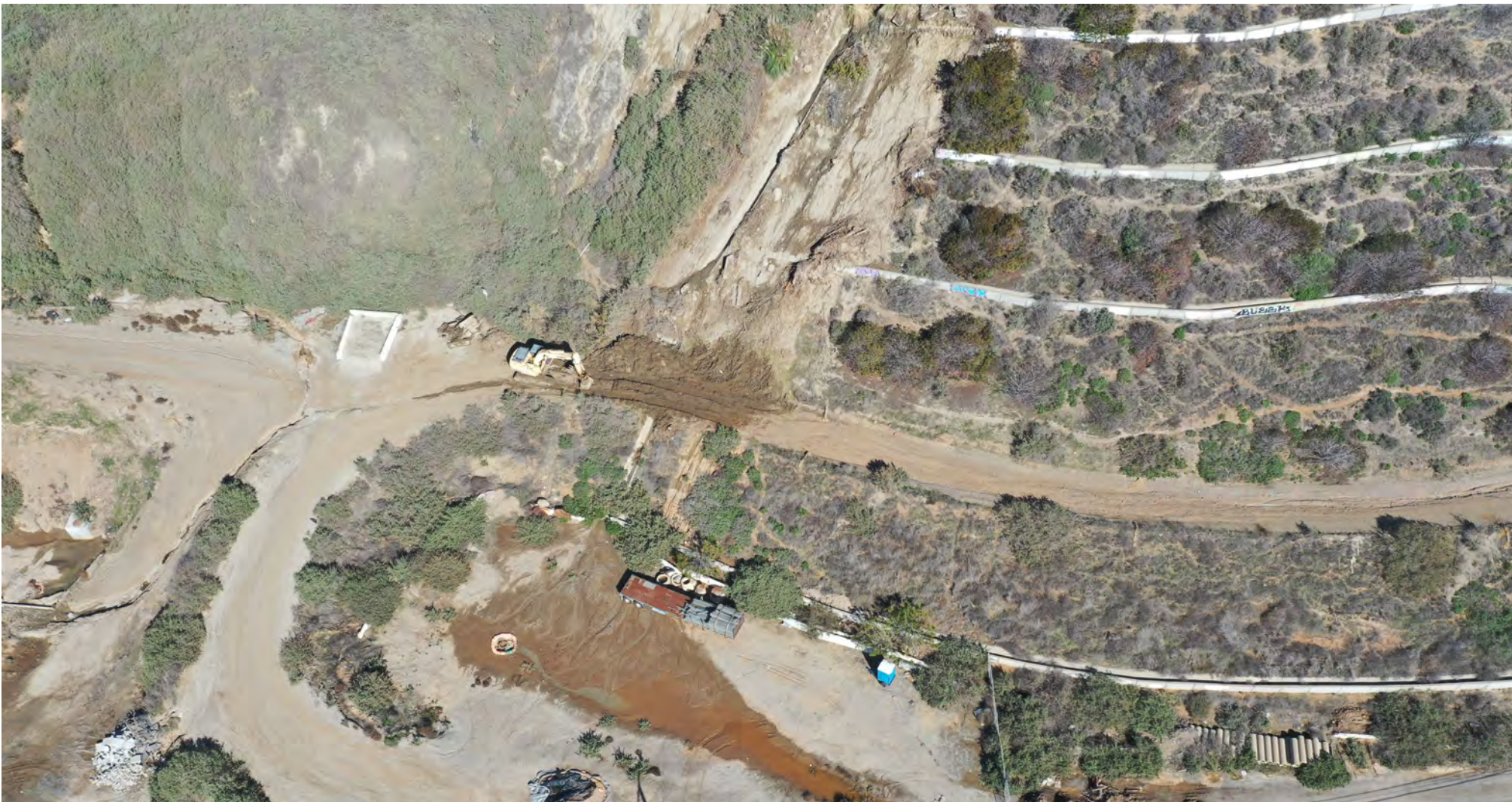
Photo 7: Looking northeast from Pacific Coast Highway. A landslide deposited mud and debris onto the access road. Severe erosional rutting also prevented access to the project stockpile as shown on the left.
