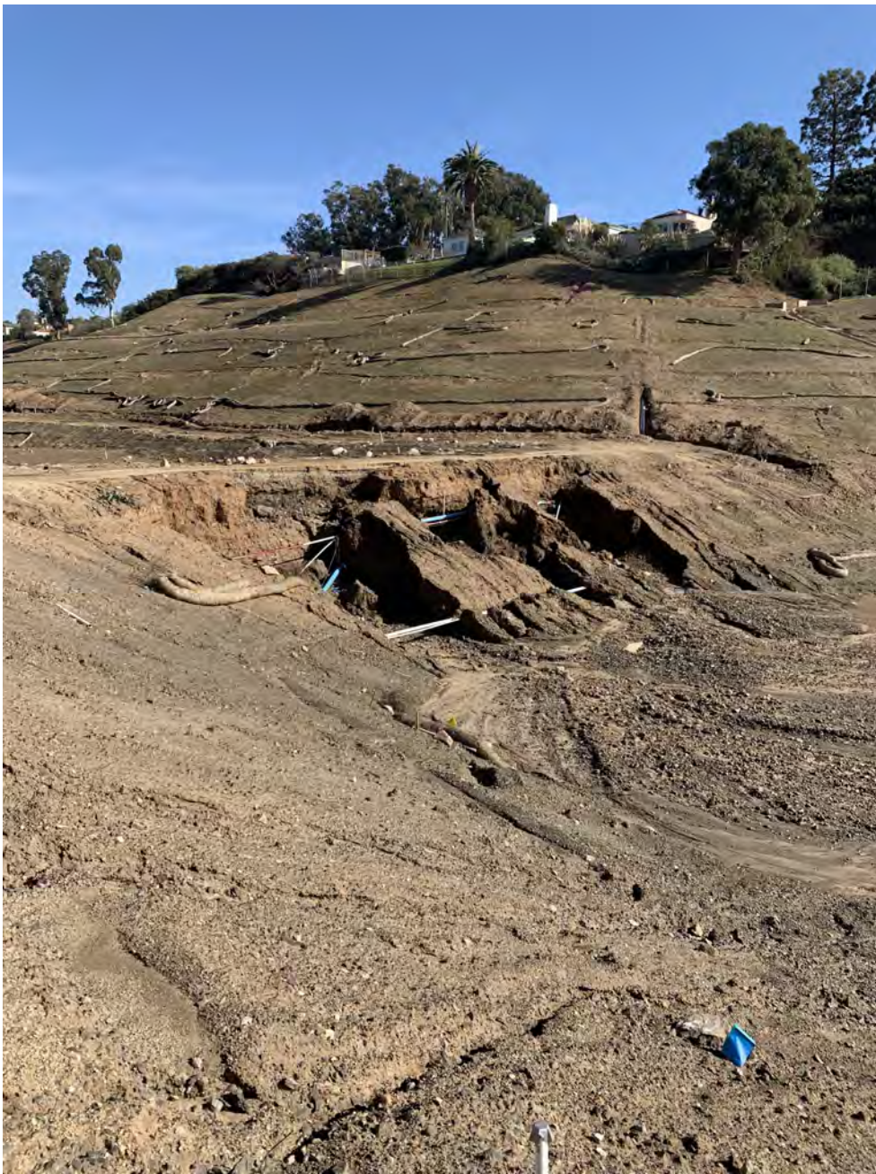
Photo 1: Looking northeast at the Basin 9 berm after the December storms. Severe erosion caused collapse of the berm and washed mud into the basin.
